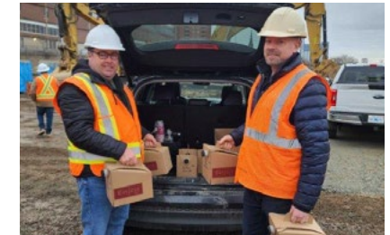
DHBC's CEO delivering coffee and treats to the Cogswell District construction team.
